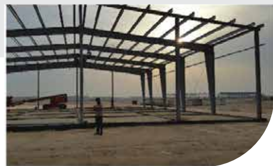
AL NEBRAS ELECTRICAL SHOP
